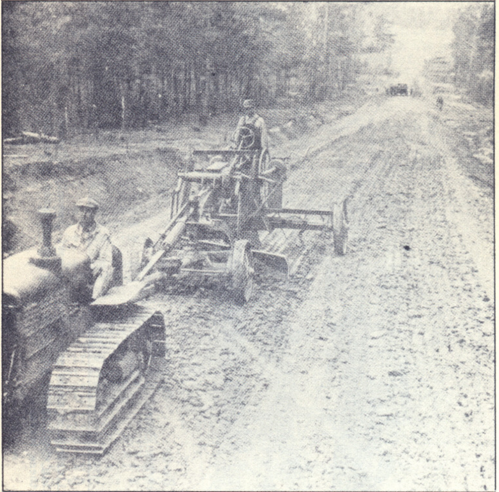
Illust. 6 -- Scarifying. When road surfaces covered with such materials as gravel and crushed stone develop chuck holes and become too rough for travel, it is necessary, usually, to scarify (rip up) the surface to the necessary depth to enable the grader to regrade and smooth up the surface again. This is because the material is too hard for the blade to cut. Here the grader is scarifying a surface for regrading.
