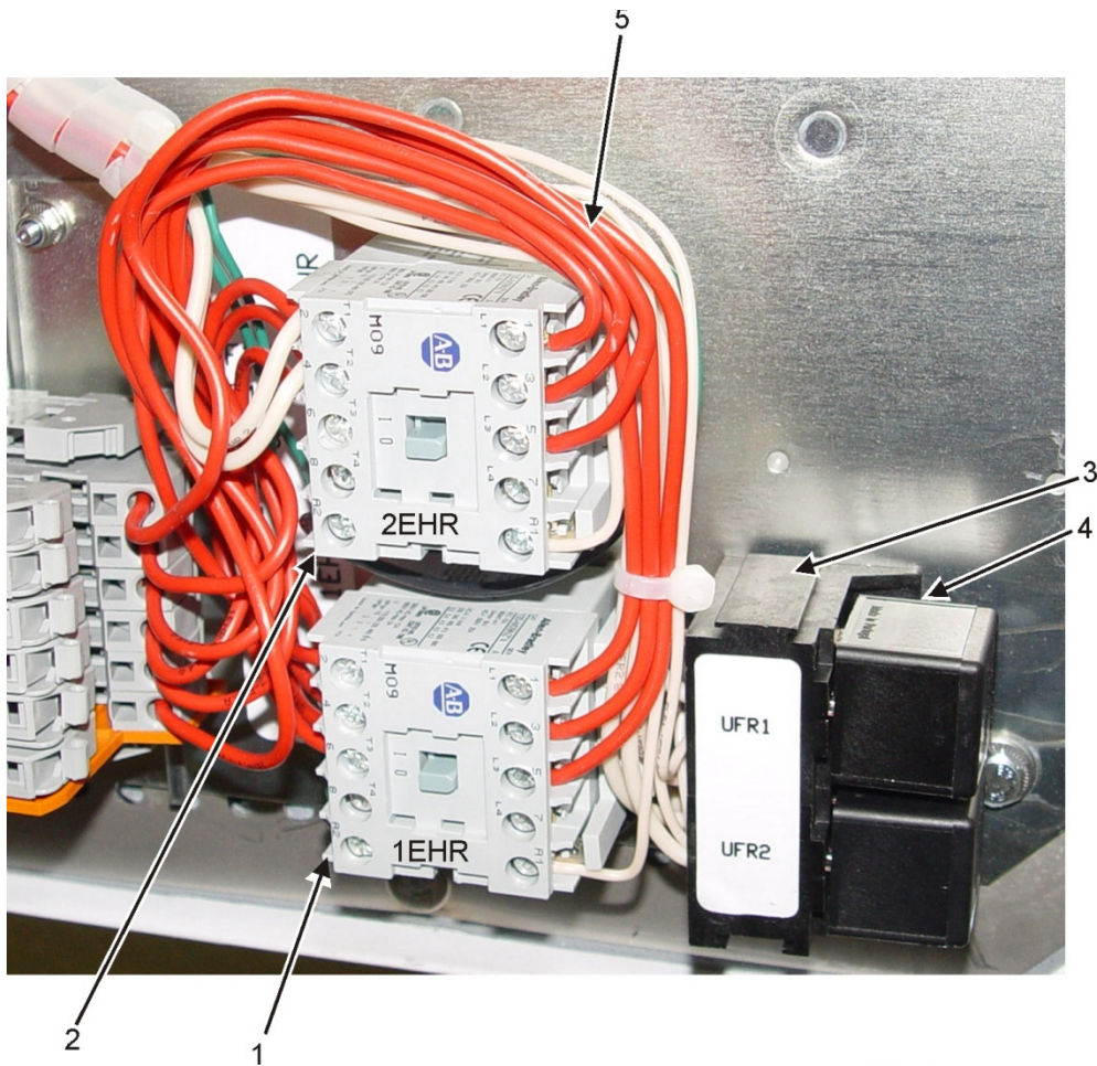
Figure 14. Evaporator Heater Relay.
