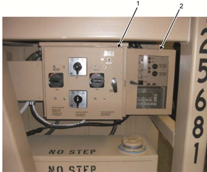
Figure 6. Power Box and Control Panel Assembly Door.
