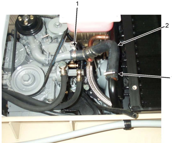
Figure 18. Water Pump Supply Hose Connect.
