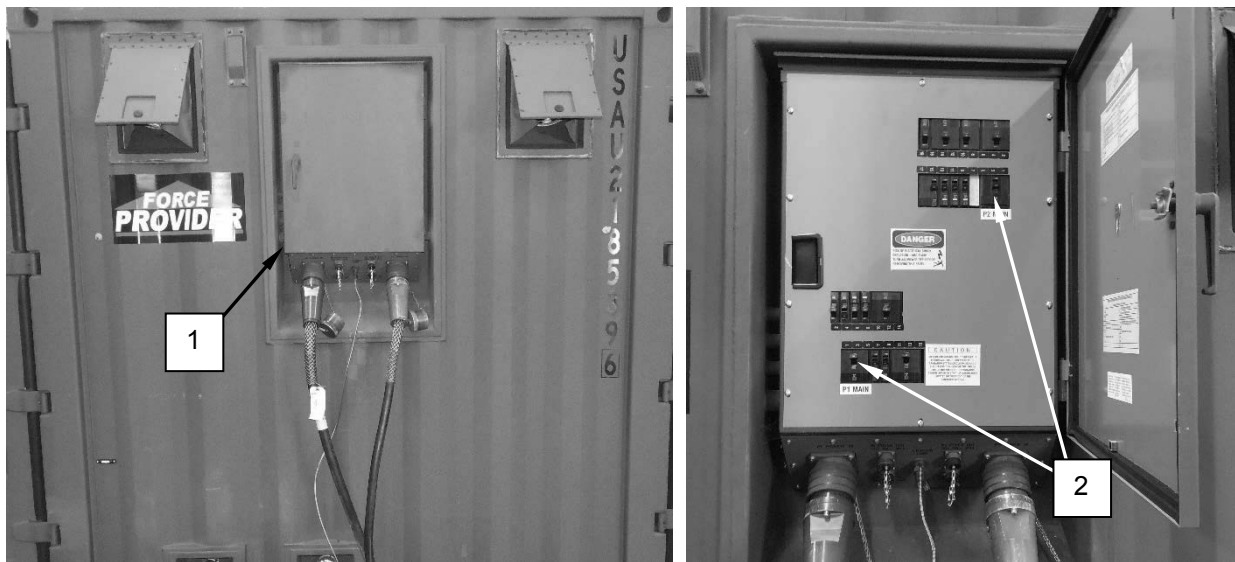
Figure 8. Reset Main Circuit Breakers.
