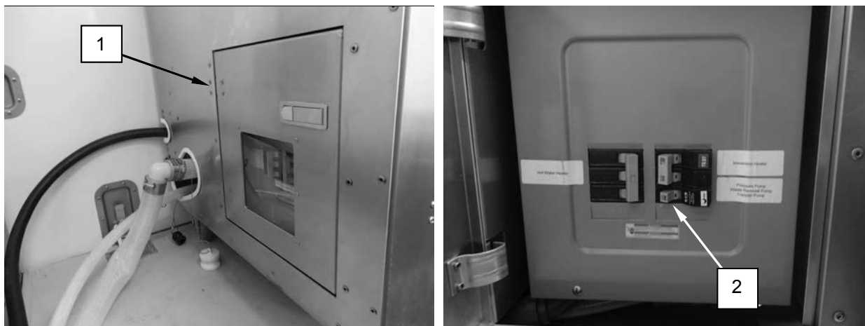
Figure 4. Resetting the Pressure Pump Circuit Breaker.
