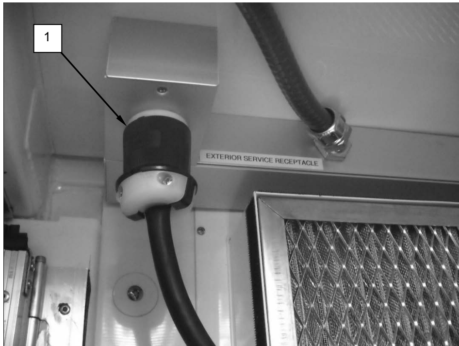
Figure 1. 50-ft Power Distribution Cable.
