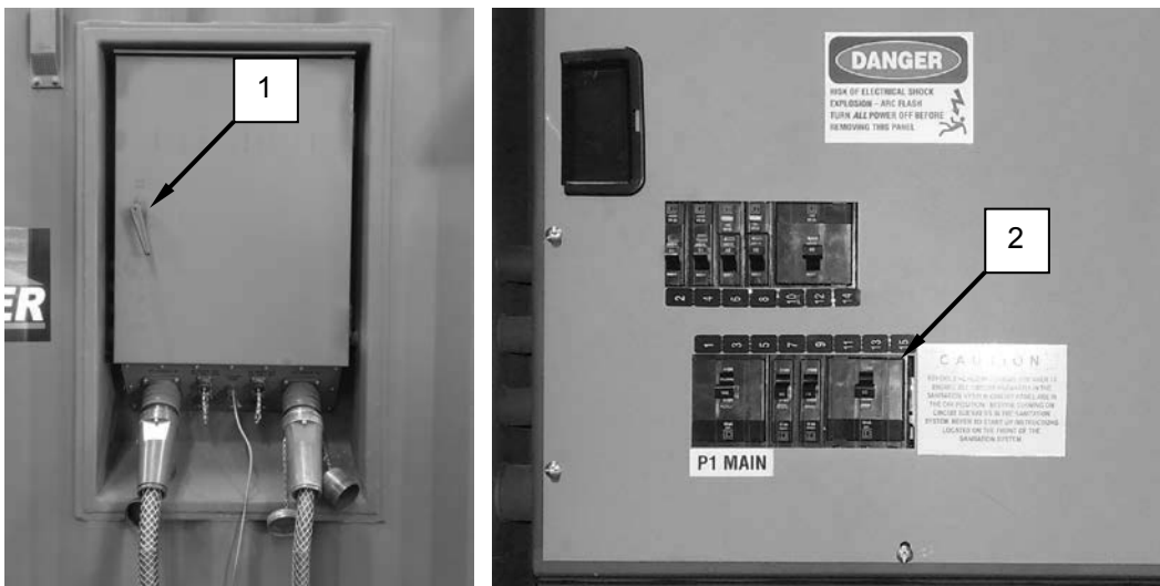
Figure 5. Sanitation Sink Circuit Breaker.
