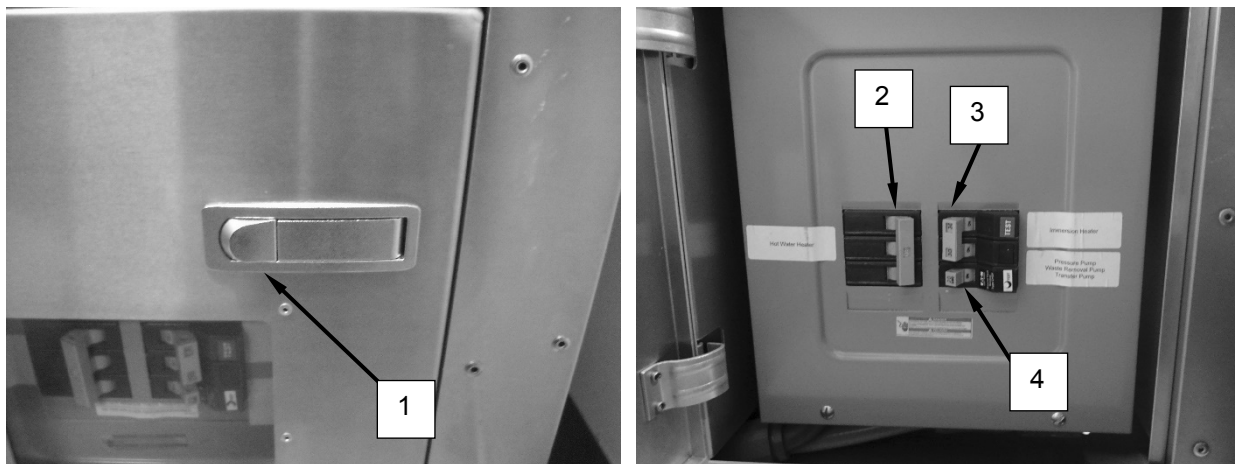
Figure 3. Sanitation Sink Circuit Breakers.
