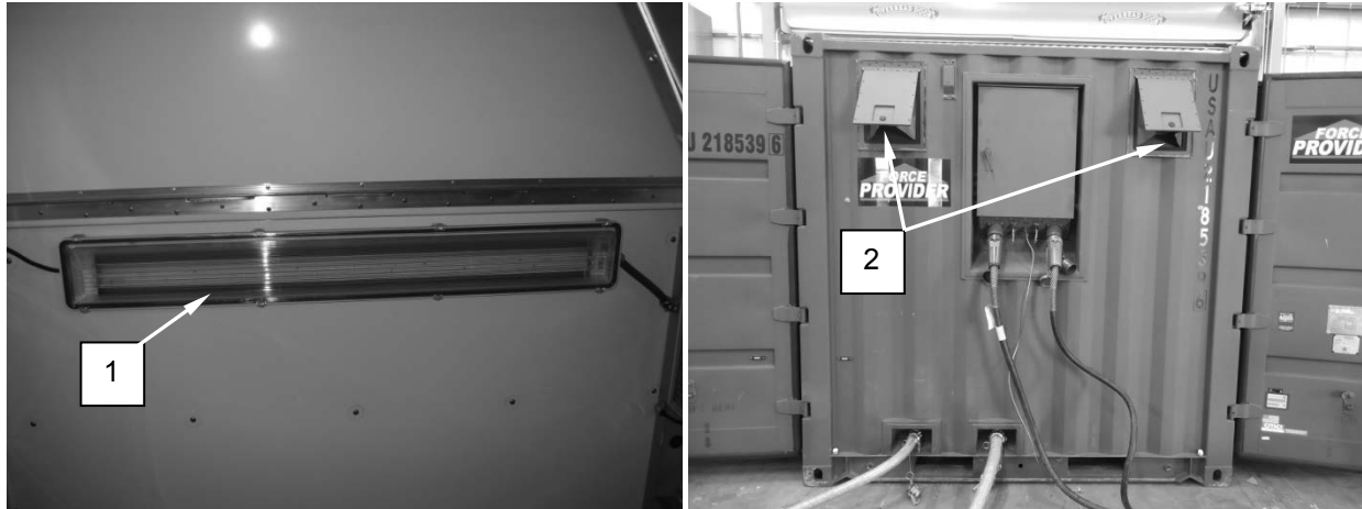
Figure 3. Fans and Lights.
