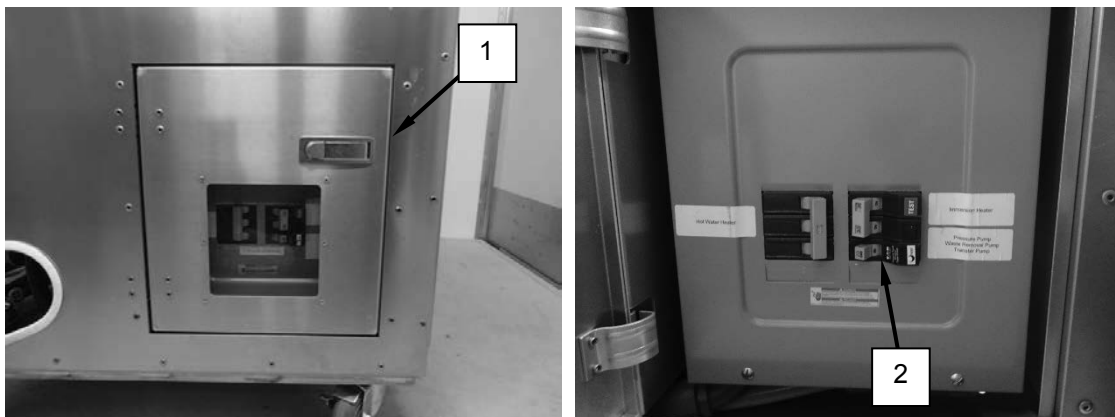
Figure 6. Sink Power Cable and Pump Circuit Breaker.
