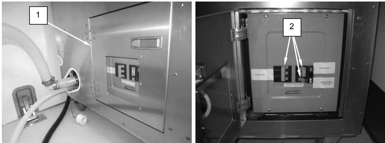
Figure 34. Verify Sink Circuit Breakers are Off.
