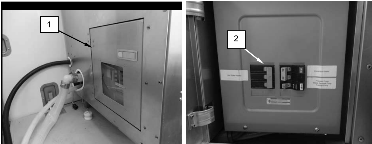
Figure 2. Resetting the Water Heater Circuit Breaker.
