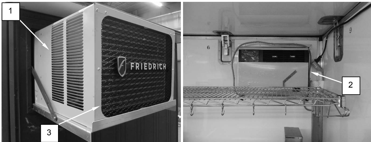
Figure 1. Air Conditioner Vents and Exhaust.
