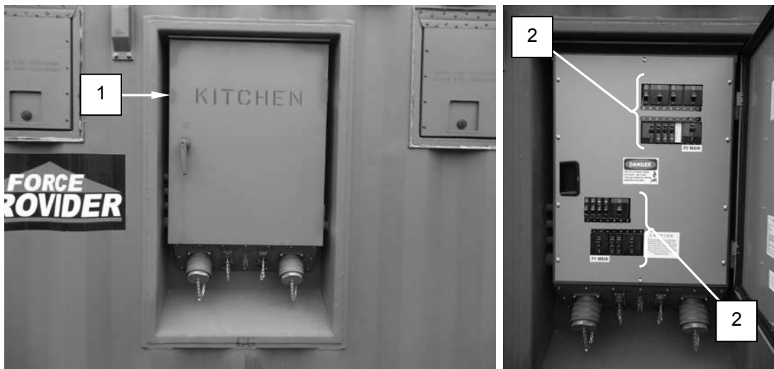
Figure 48. Circuit Breaker Panel.
