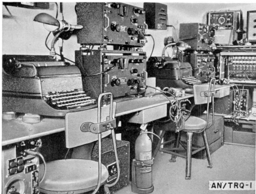
Figure 29. Radio Control Central AN/TRQ-1 installed in Shelter HIO-17.
