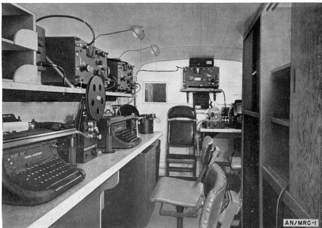
Figure 11. Radio Set AN/MRC-1, components installed in shelter.
