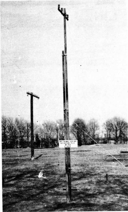
BRITISH MAL-EXTENSION POLE WITH WIND STAYS
