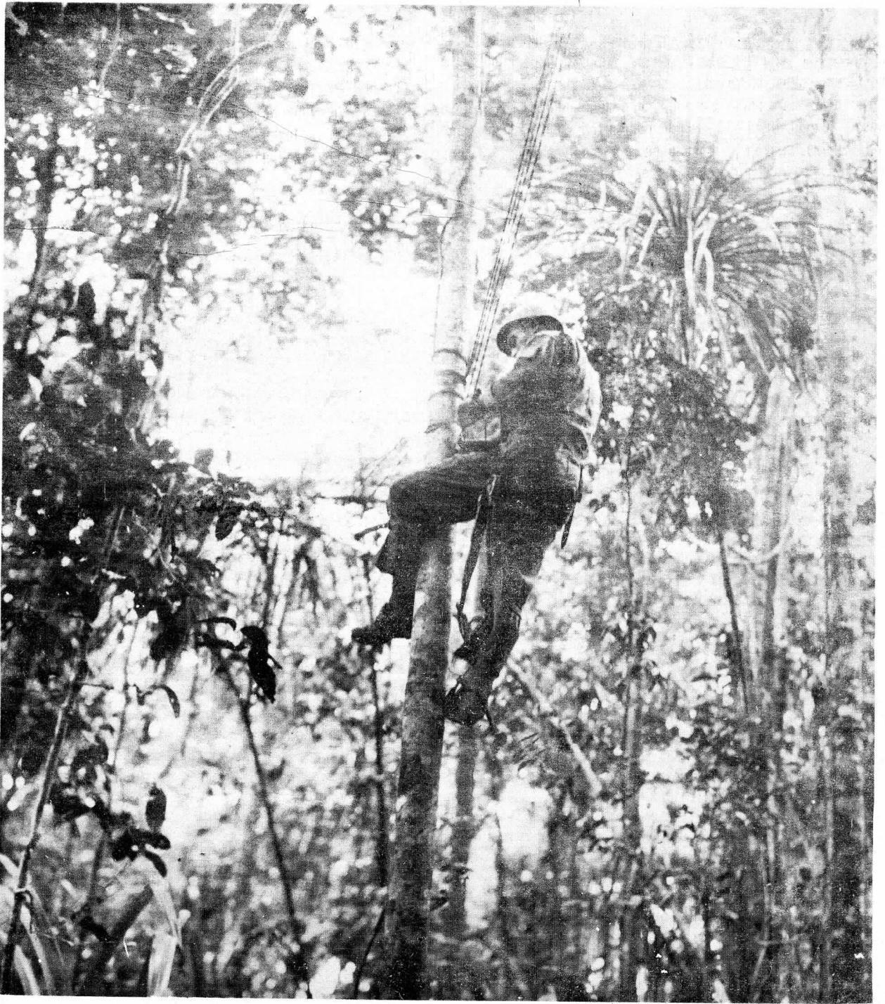
"WHEN TIME PERMITTED ALL CIRCUITS-----WERE FASTENED FROM SEVEN TO TWENTY FEET OFF THE GROUND TO CLEAR TROOPS AND VEHICLES." HERE NATURE SUPPLIED THE POLES.
