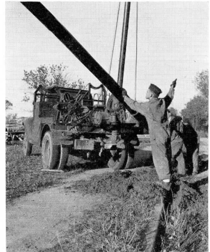
The hole was drilled by an automatic digger but it takes the human eye to set a telephone pole straight
