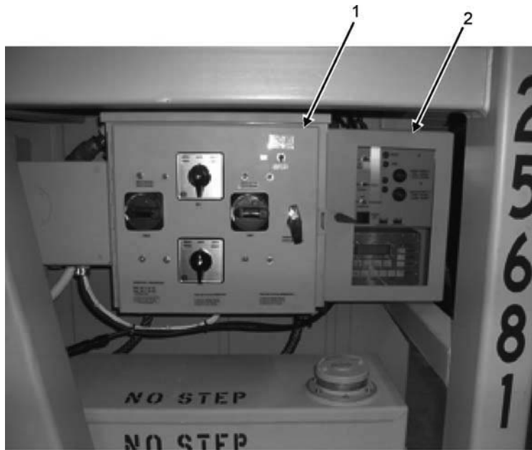
Figure 5. Power Box and Control Panel Assembly Door.
