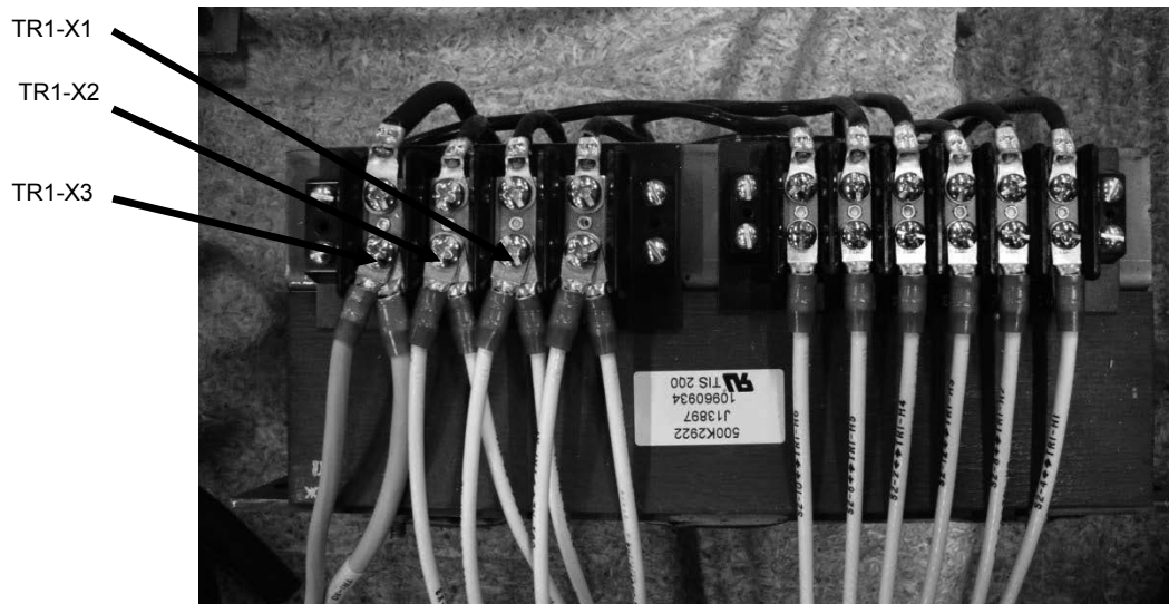
Figure 6. Transformer Terminal Block.
